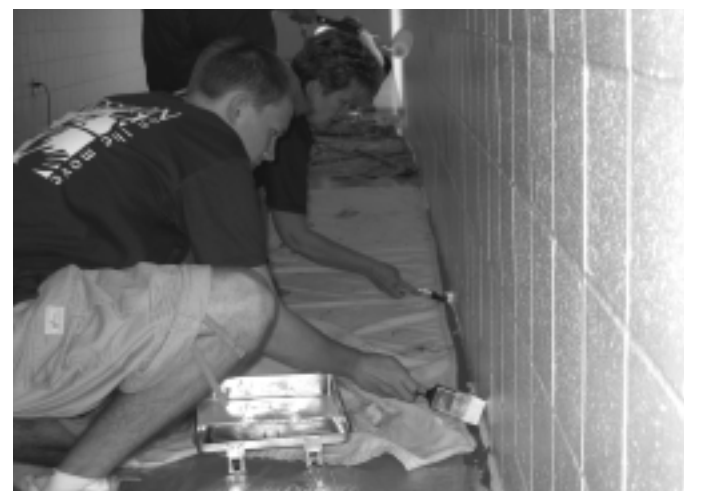
Joan McCleish, Mercy College, and her son, Steven help paint the Wellness Center located in the John R. Grubb YMCA facility.
